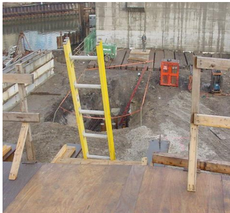
Unprotected Open End
